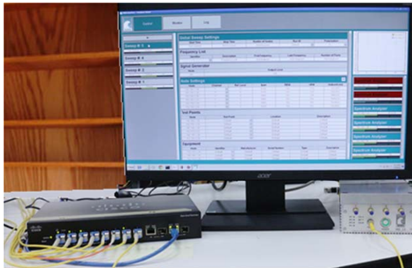
Figure 2: CWI-Net 2.0 Control GUI, 8-port fiber optics Ethernet switch, and node interconnected.
